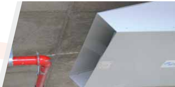
Figure 10(d). Pipe work can impede fan throw
