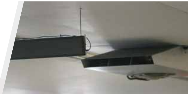
Figure 10(b). Warning signs can impede fan throw
