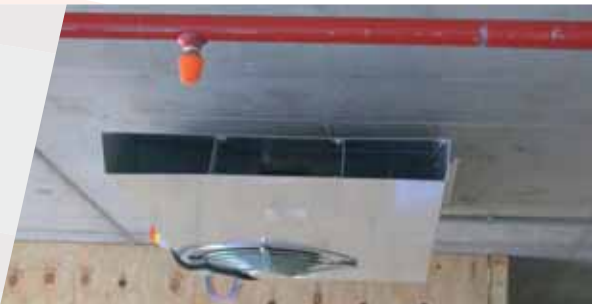
Figure 10(c). Clashes with sprinkler heads can impede fan throw
